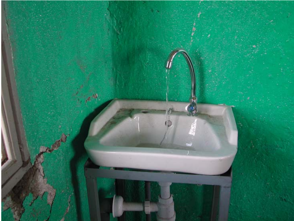
Photo 7. Sink for hand washing installed in the clinic
