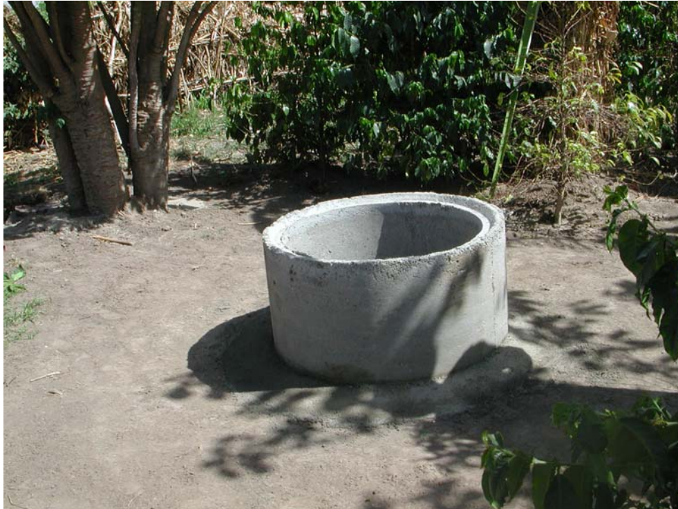
Photo 10. View of the hand dug well of Ato Bulema after masonry work and installation of concrete ring
