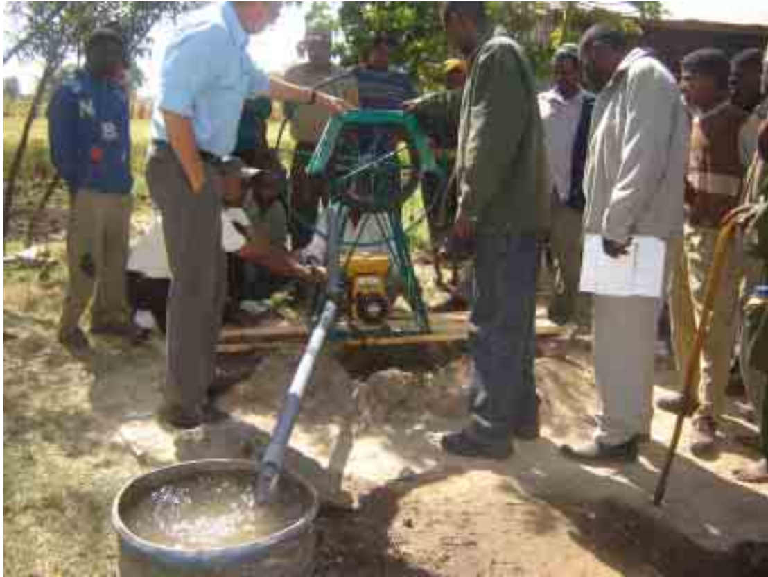
Figure 62: Motorized (diesel motor) rope pump demonstration
