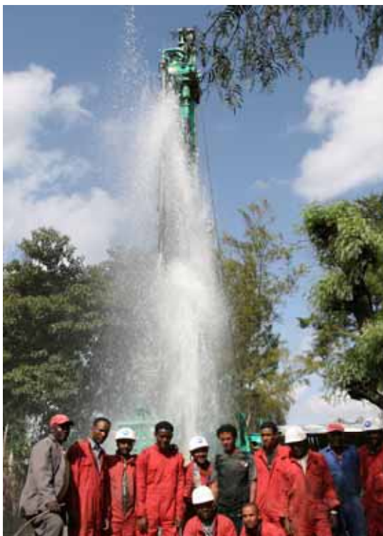
Providing water to a community in the town of Inseno through the Butajira-Ziway Development Program
